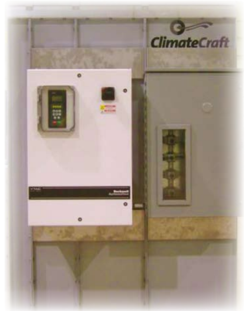
VFD Control Panel & Power Distribution Panel
