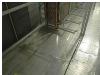
Double sloped drain pans
