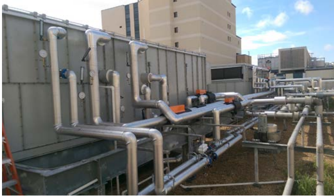
Halifax Medical Center Daytona Beach, Florida Two custom air handlers and two ACCESS site-assembled air handlers
