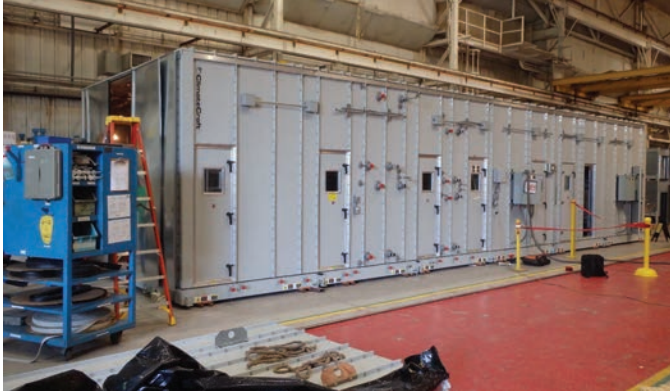
Air handler undergoing pressure testing in the factory
