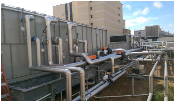
Halifax Medical Center Daytona Beach, Florida Two custom air handlers and two ACCESS site-assembled air handlers
