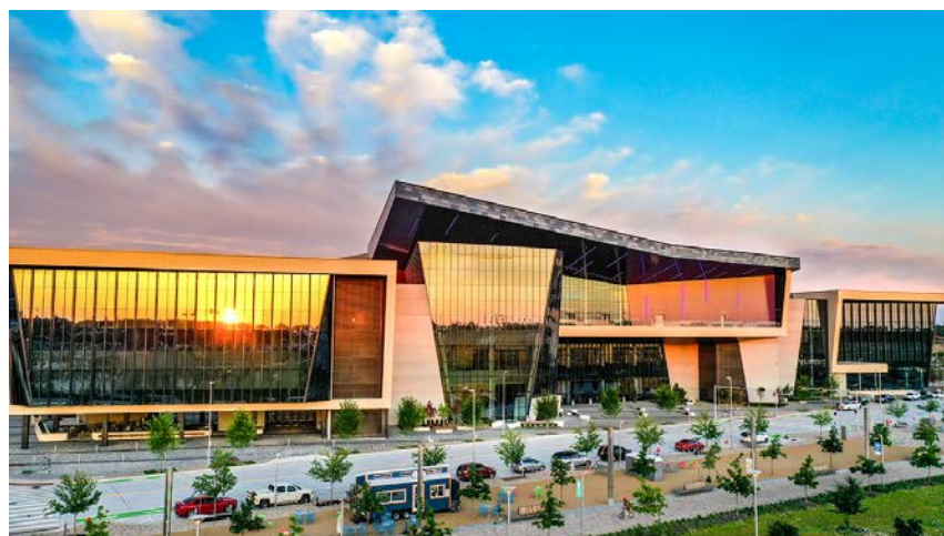
Convention Center Oklahoma City, Oklahoma 28 custom air handlers and one makeup air handler
