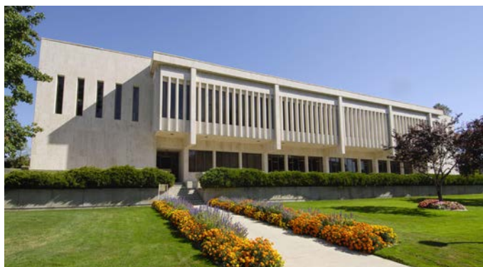
Idaho State Supreme Courthouse Boise, Idaho One ACCESS site-assembled air handler
