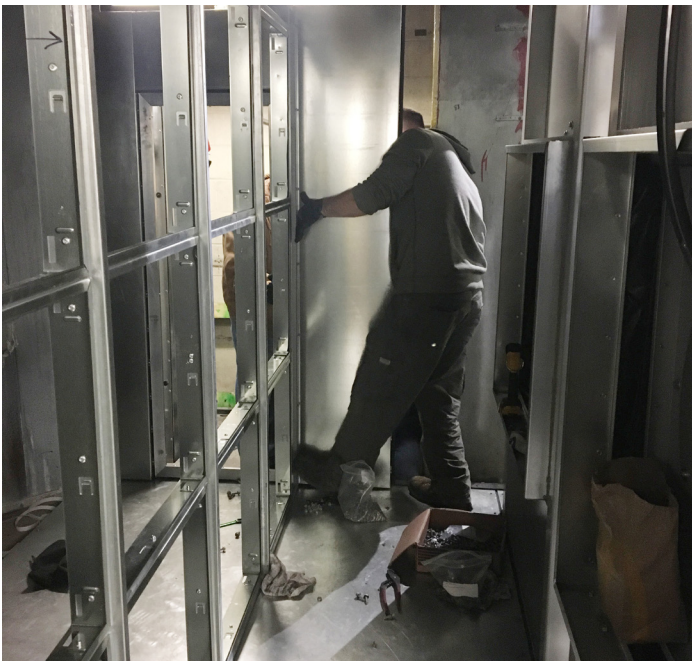
Assembling the panels on the framework of the ACCESS air handling unit
